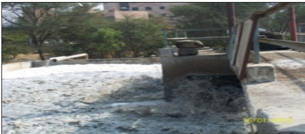
Fig.-2: Effluent (Aeration Tank) Jaipur Dairy
